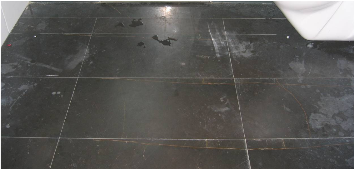
Above picture shows acid etching (dull drip marks from acid used to clean wall tiles)
